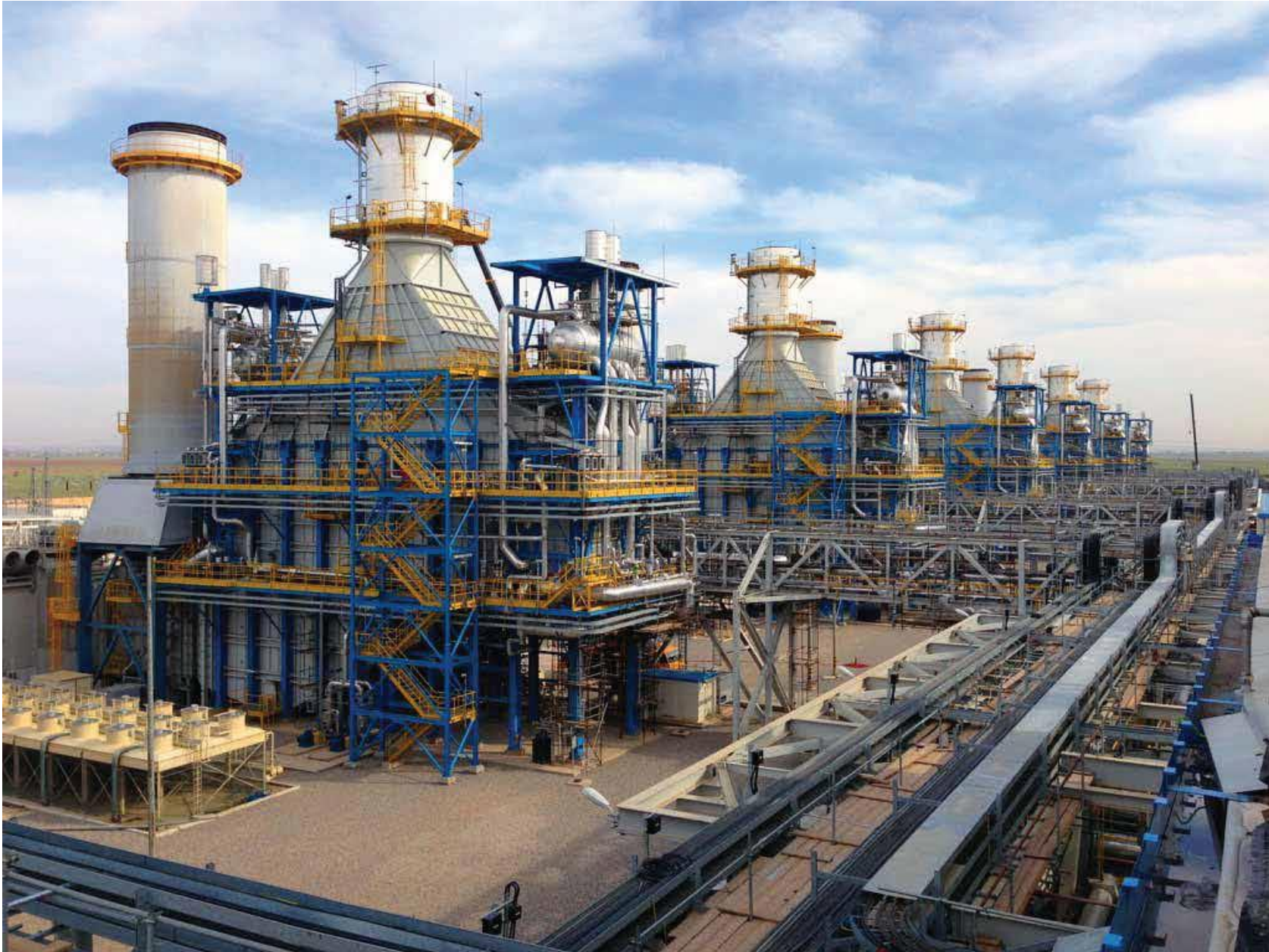
ERBIL POWER PLANT
