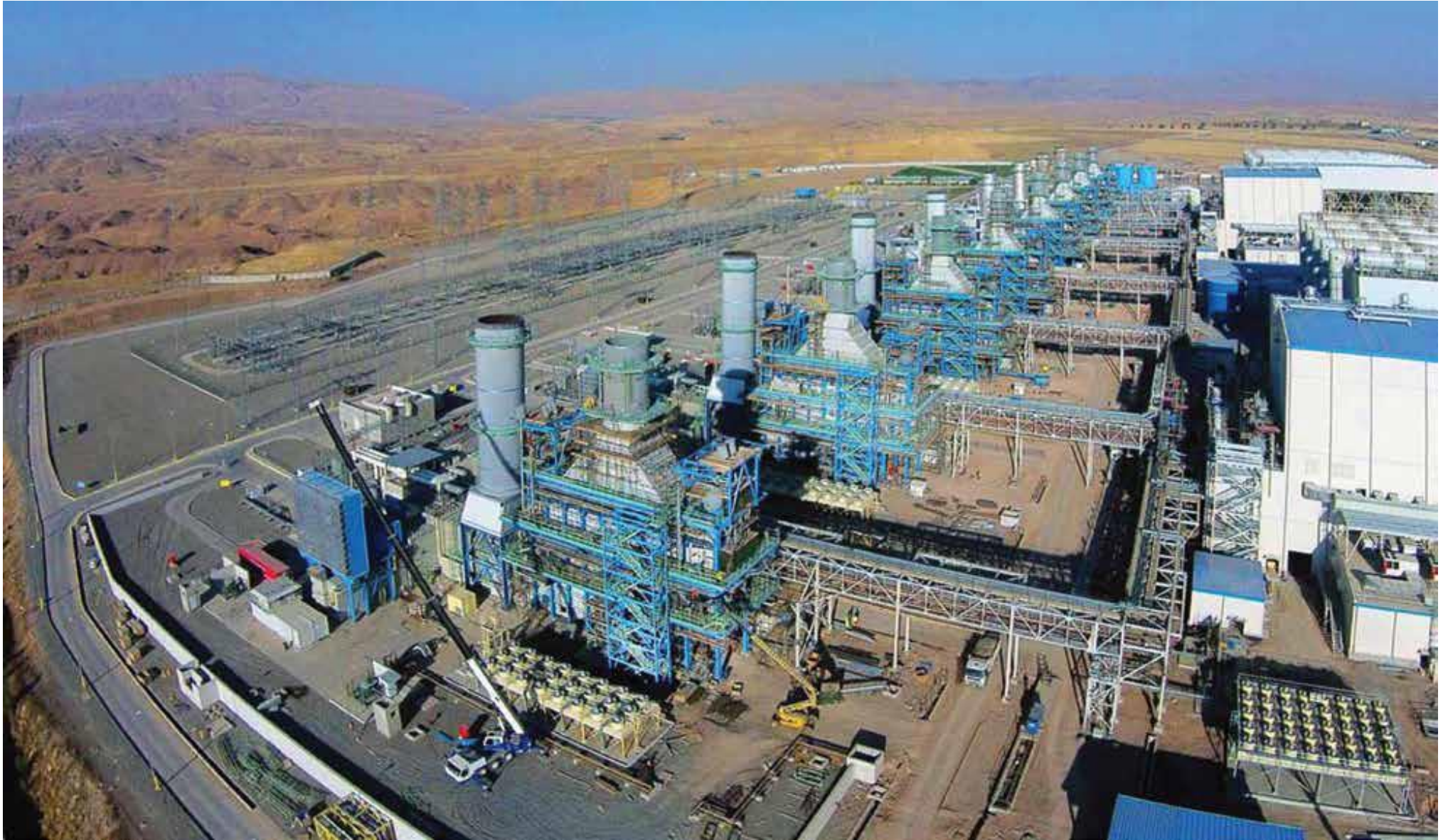
SULAYMANIYAH POWER PLANT
